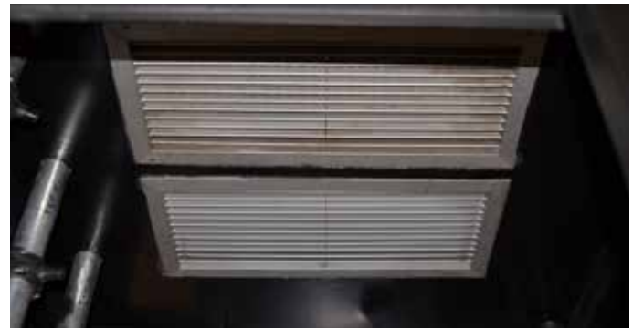
Top entry intake air louvres provide a shower effect
